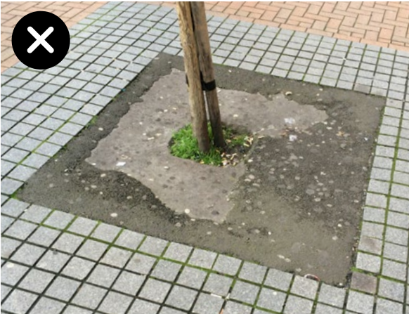
Poor example of asphalt application
