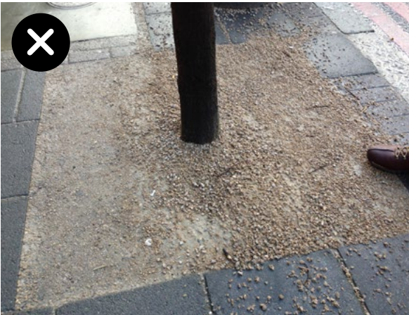
Poor example of self-binding gravel application
